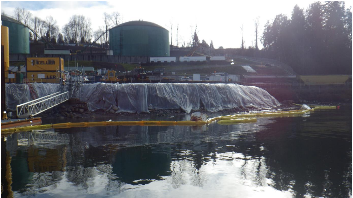
Photo 2. Polysheeting that will be replaced with coco matting to reduce erosion.
