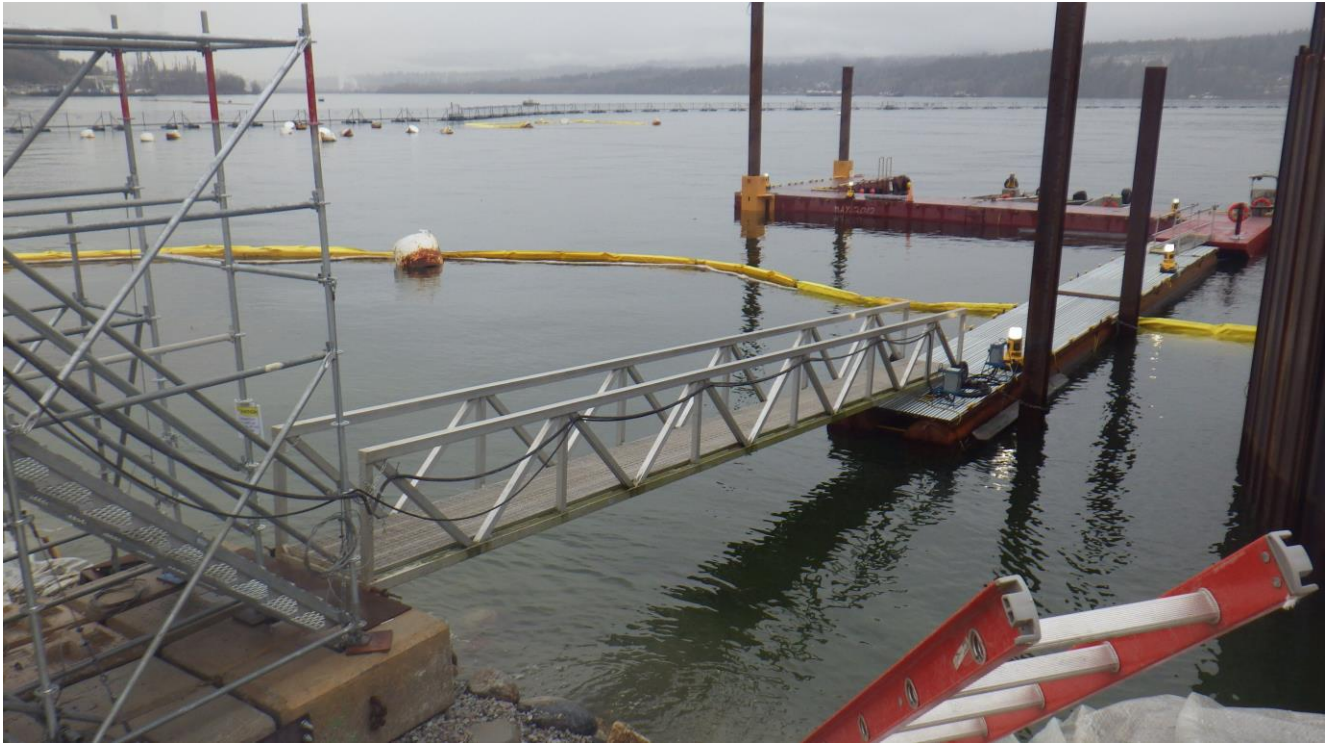
Photo 1. Gangway and flexi-float dock constructed to replace small utility dock and will be removed after marine construction office is built.
