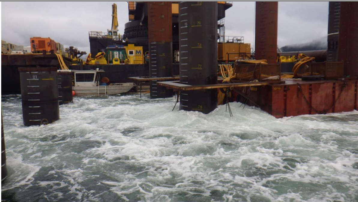
Photo 4. Activated bubble curtains, which are used to dampen underwater noise levels during impact pile driving, being tested in the absence of impact hammer pile driving.
