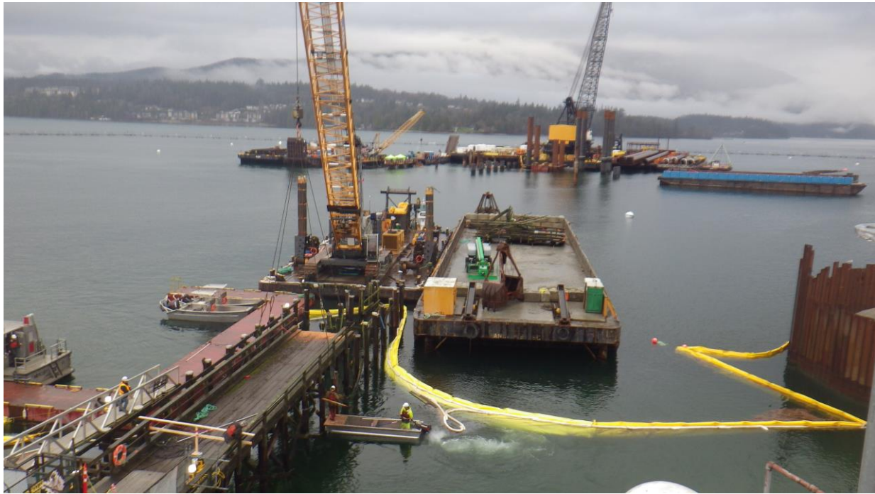
Photo 1. Yellow turbidity curtain and white sorbent boom installed around utility dock during dock demolition activities conducted by JJM.
