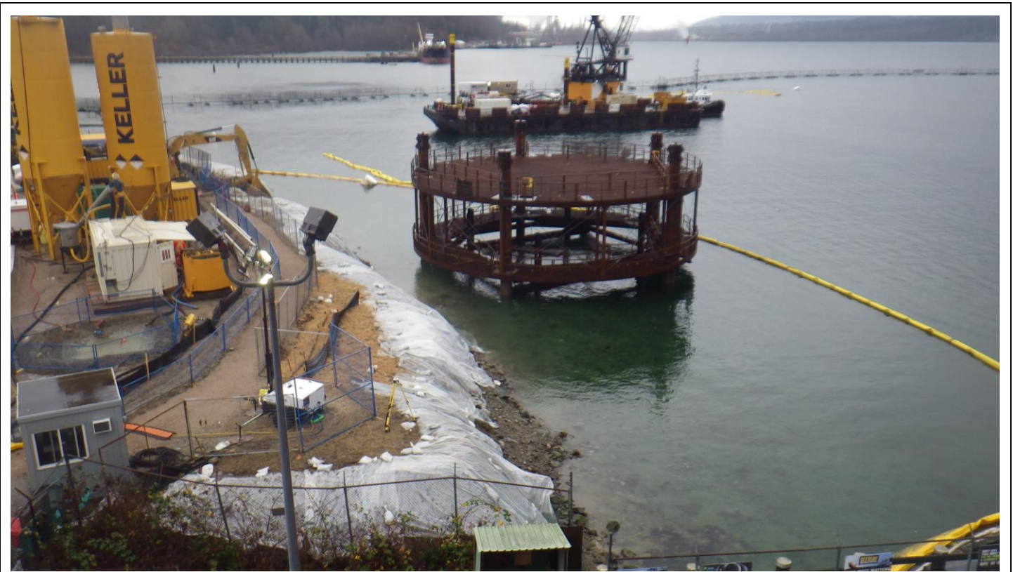
Photo 3. Yellow turbidity curtain around works associated with installation of temporary flexi-float dock.
